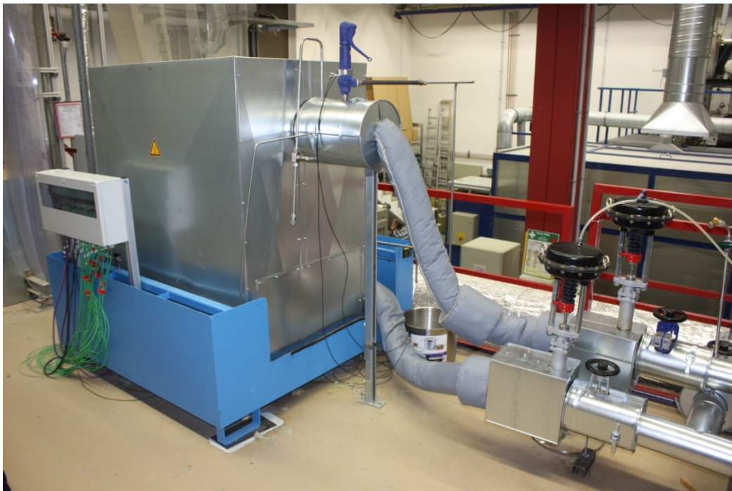
Fig. 2: Insulated experimental setup of DLR's flat plate latent heat storage
