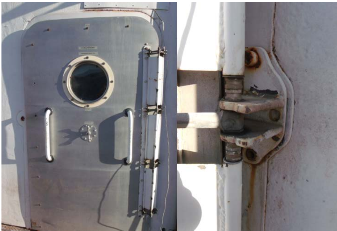
Figure 5: Left picture: The closed outer engineering airlock door. Note the hinges on its right side and the lack of support on its left side. Right picture: One of the bottom hinges. It is strongly constructed, but decay and probably dynamic forces made it loose a screw.
