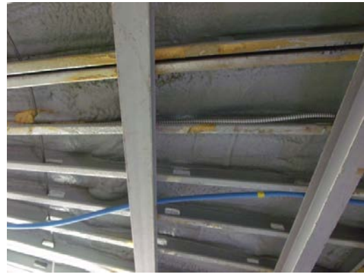
Figure 3: MDRS interior floor beams in 2013, note the slightly rusty spots.
