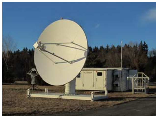
Figure 2 TM Station with Antenna
