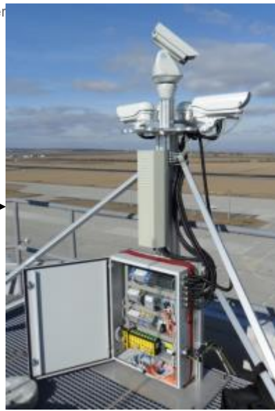
Cameras on top of the Tower Erfurt
