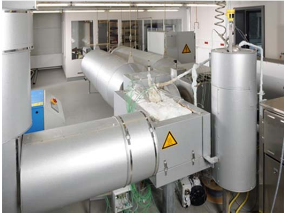
Figure 2. Multifunctional pilot plant for thermo-chemical storage reactors
