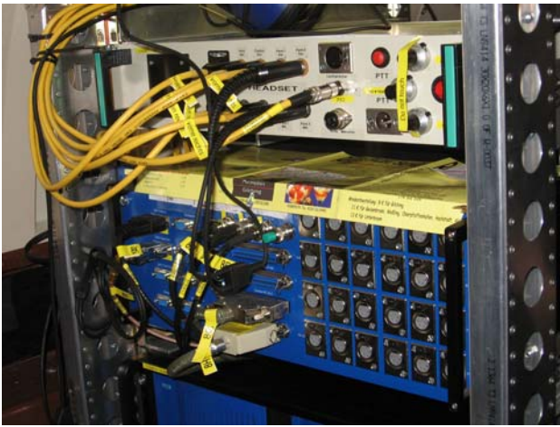
Figure 16 Auxiliary Rack: Intercomm, Breakoutbox, ALC control PC, Multi Input Recorder PC.
