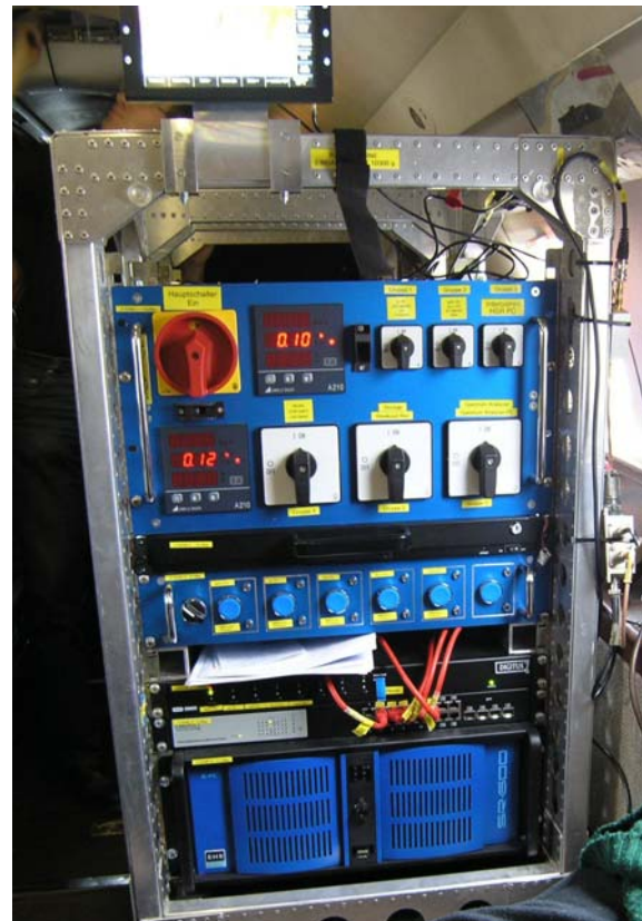
Figure 15 Operators rack: Power distribution box, Monitor drawer, PC start box, KVM switch, network switch, Operators PC.
