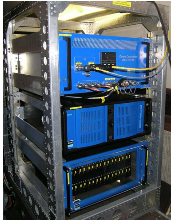
Figure 14 HSR rack: RF Frontend, Highspeed Recorder PC, Data Storage (32 disks).
