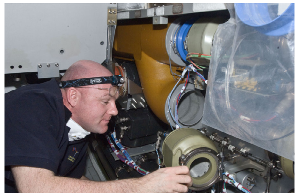
Fig. 3: André Kuipers during inspection and cleaning of the CFA ducts (Credits: NASA)
