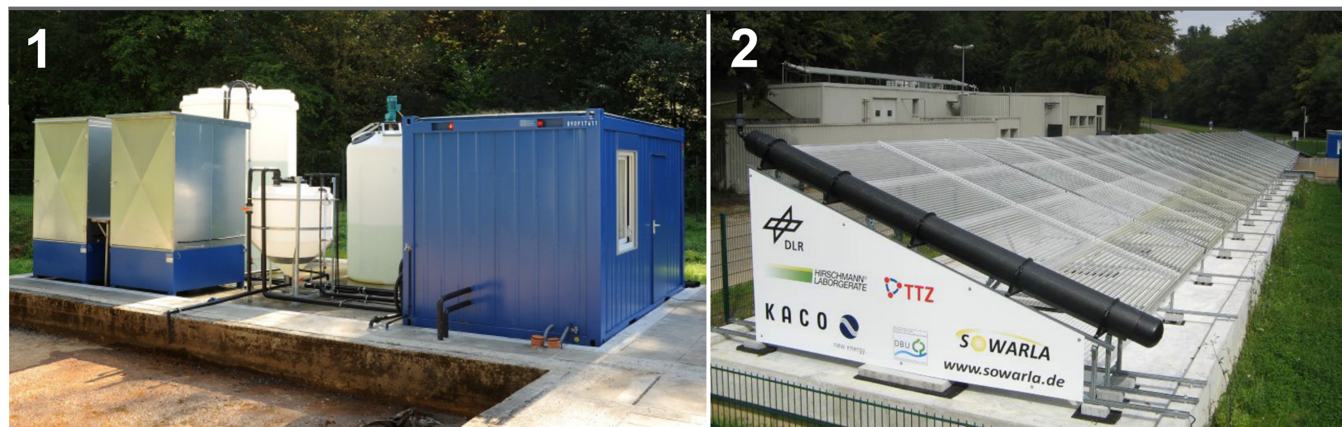
Figure 1: Solar water treatment plant at DLR's Lampoldshausen site, Germany. (1: fluid system with recirculation tank, photocatalyst recycling system and storage tanks; 2: tubular receiver reactor)
