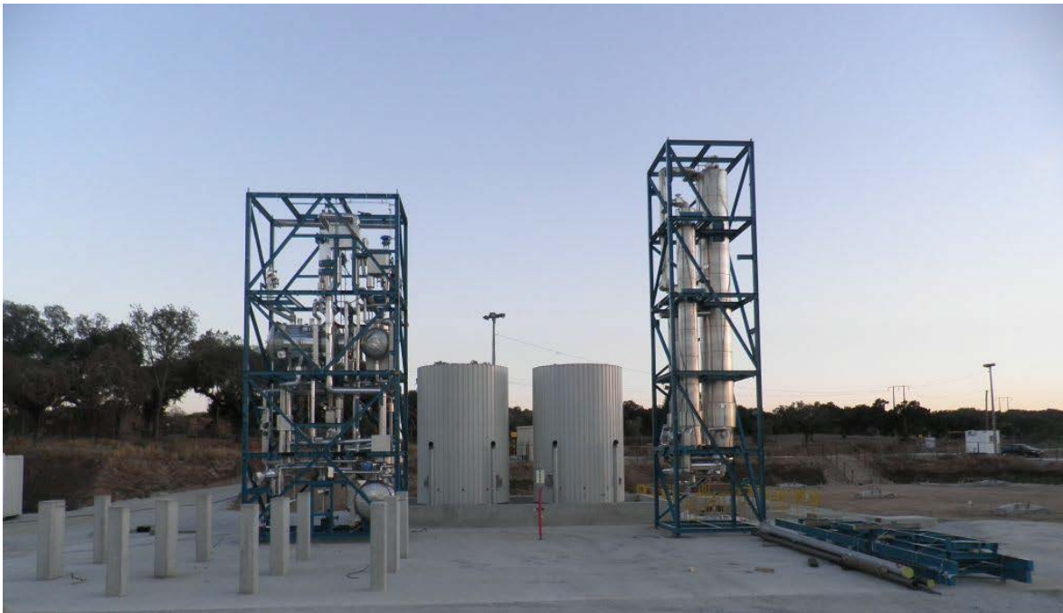
Fig. 3: Steam generating system (skid on the right side) and water cycle (skid on the left side) with high live steam design parameters of 580 °C and 140 bar
