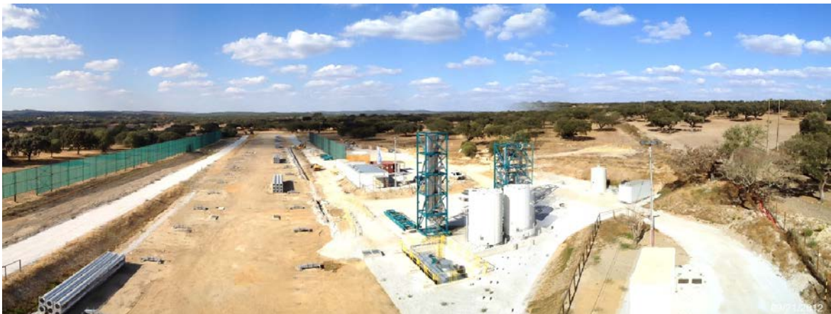
Fig. 2: Panoramic view of current status of the construction site. On the left hand side the solar loop will be erected. The drainage tank is shown on the lower center, the two storage tanks are show on the right hand side and the two blue skids contain the SGS and the water cycle
