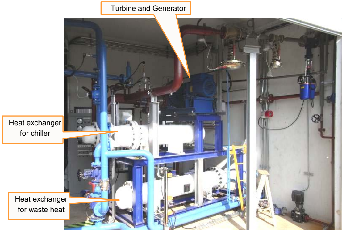
Fig. 4. Turbine with generator and condenser
