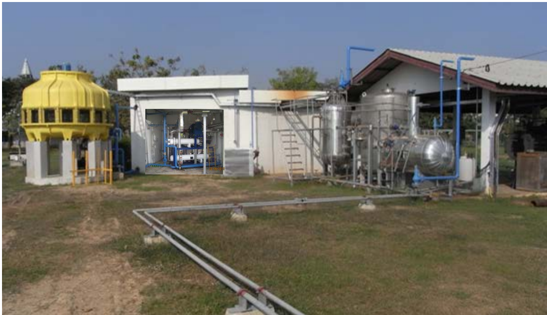
Fig. 3. General view of the power block. Left: Cooling tower. Middle: Turbine and condensators. Right: Steam drum and feed water tank
