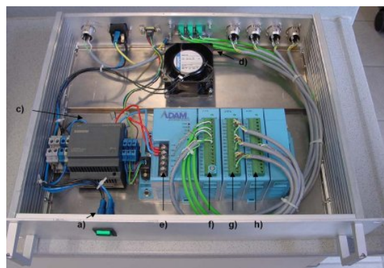
Fig. 4. Data acquisition system
