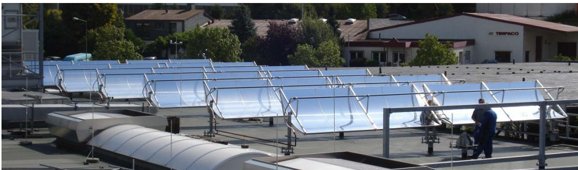
Fig. 1: Solar field with PTC1800 parabolic trough collectors
