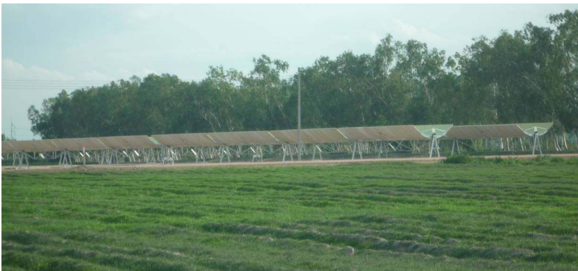
Fig. 2. Collectors at the KTSE-9100 Power Plant
