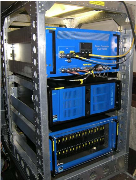
Figure 14 HSR rack: RF Frontend, Highspeed Recorder PC, Data Storage (32 disks).
