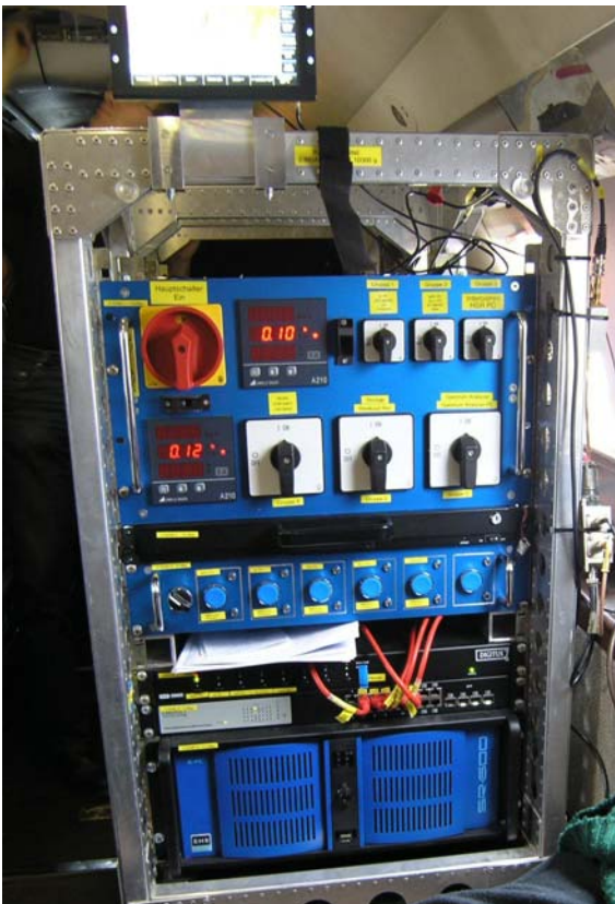
Figure 15 Operators rack: Power distribution box, Monitor drawer, PC start box, KVM switch, network switch, Operators PC.
