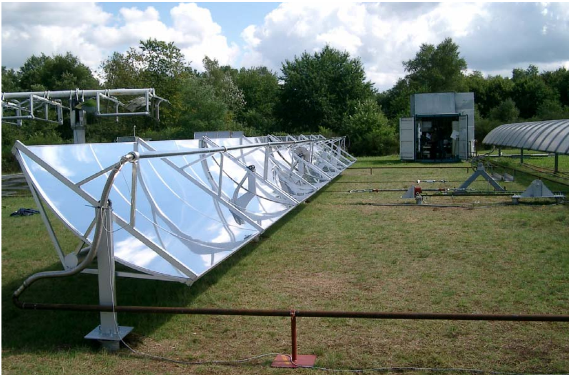
Fig. 1: SOLITEM PTC 1800 collector at DLR testfacility, Cologne
