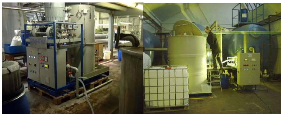
Figure 2: PhoRTex lamp driven 500 l by-pass plant Augsburg, Germany and 3 m 3 demonstration plant Gera, Germany
