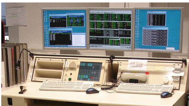
Figure 3: A typical console workplace with three monitors on two computers. Also visible is the Voice intercom touchscreen.
