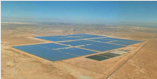
Fig.1. The 30MW SEGS III-VII parabolic trough plants in the California desert.
