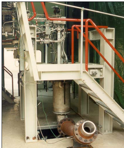
Fig. 2: Steam Generator Mode
