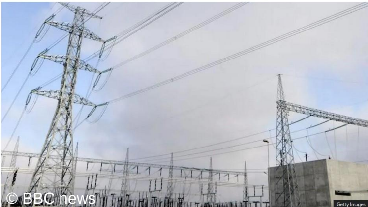
Eatlink 2 transformer station in Porvoo, Finland
