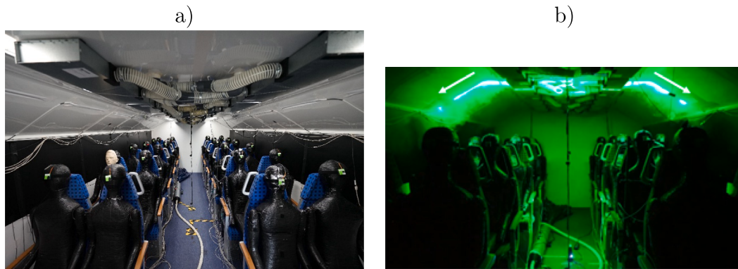
Fig. A.12. (a) Slot diffusers as supply air inlets mounted below the ceiling (as also for Sc1). (b) Laser-smoke visualization of the inflow provided by concept Sc3.
