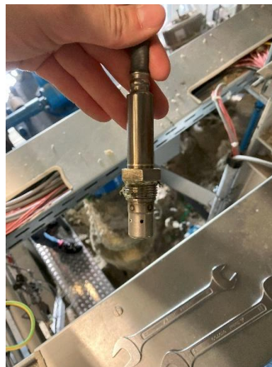
Figure 3: Sensor element placed in the gas conduit.
