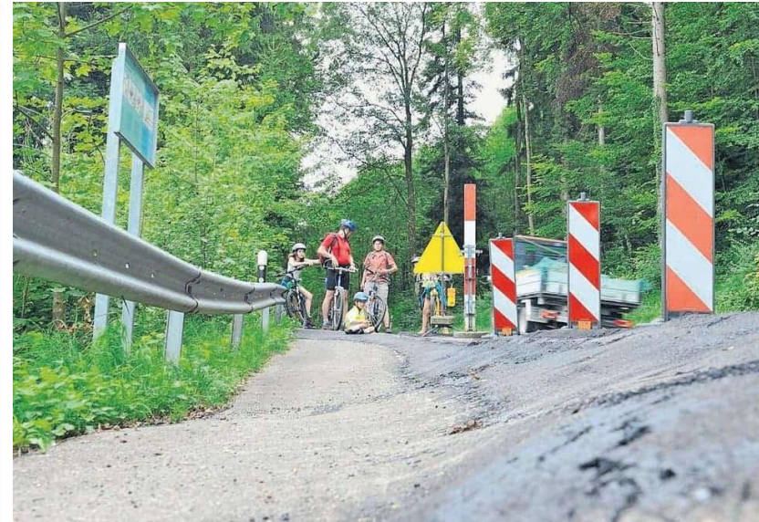
Switzerland road deformation
