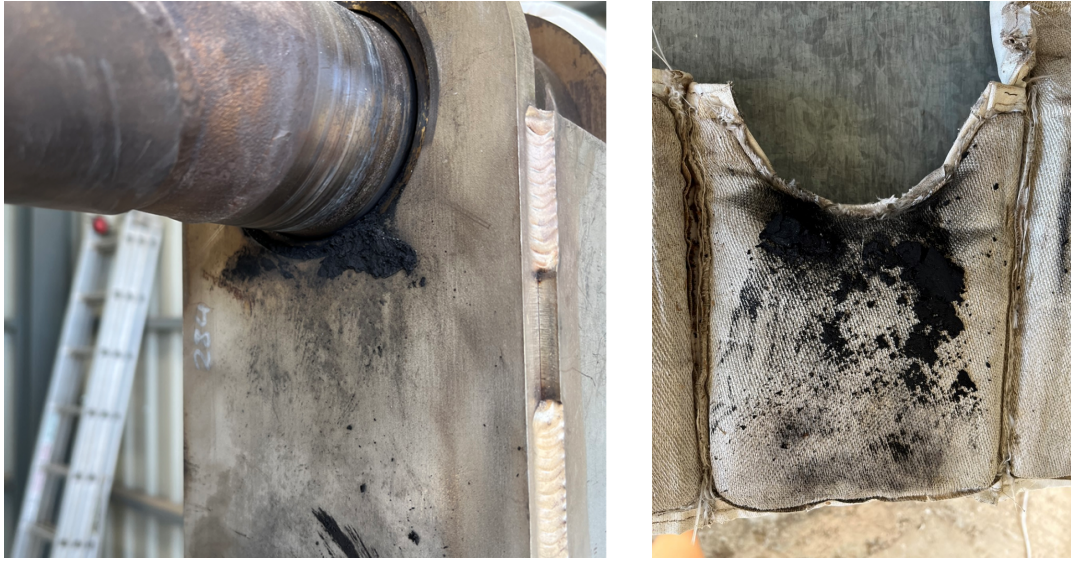
Figure 5.15.: East facing side of west swivel joint and inside of insulation after leakage
