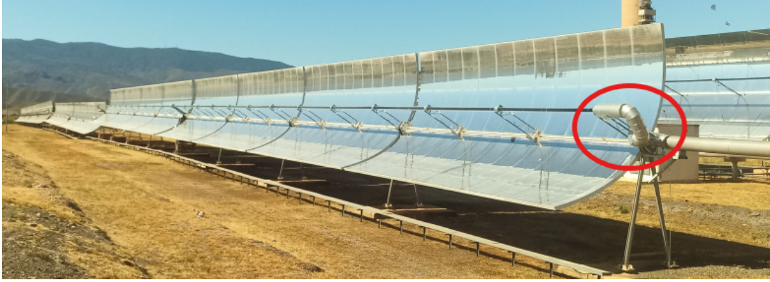
Figure 1: Series of PTCs each with parabolic-shaped mirror, mounting structure, and receiver tube. The REPA connecting the tube to the field pipes is marked.
