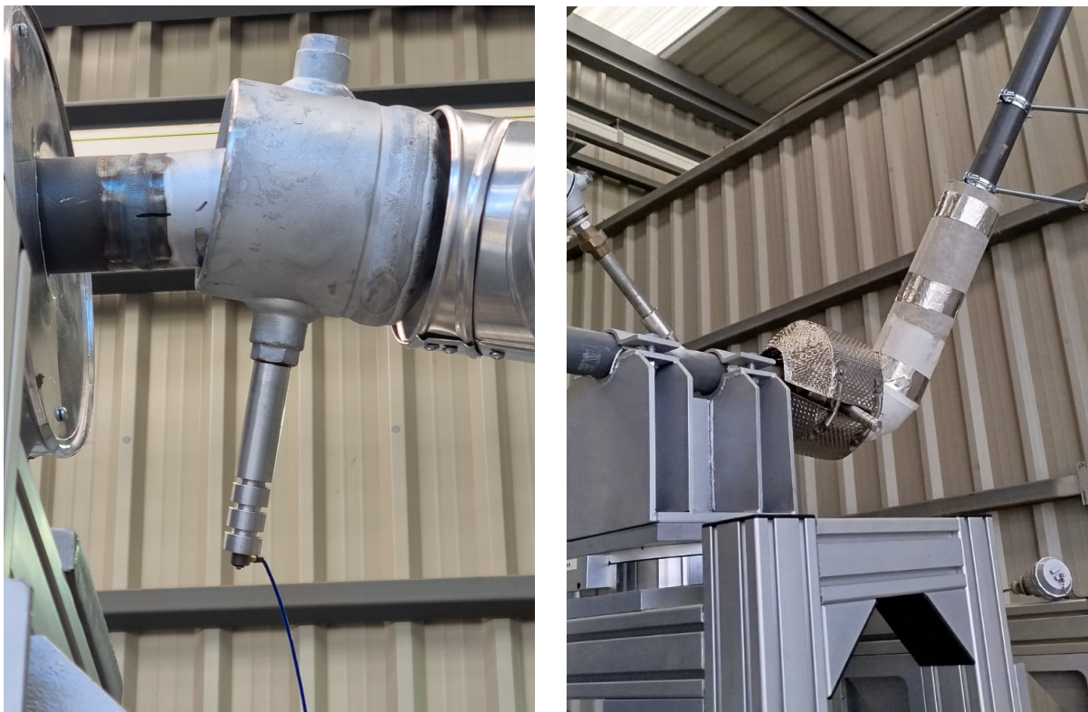
Figure 3.5: Left: Lowest ball joint with attachment for the vibration sensor and the vibration sensor installed, Right: Lowest ball joint with attachment for the vibration sensor and isolation installed
