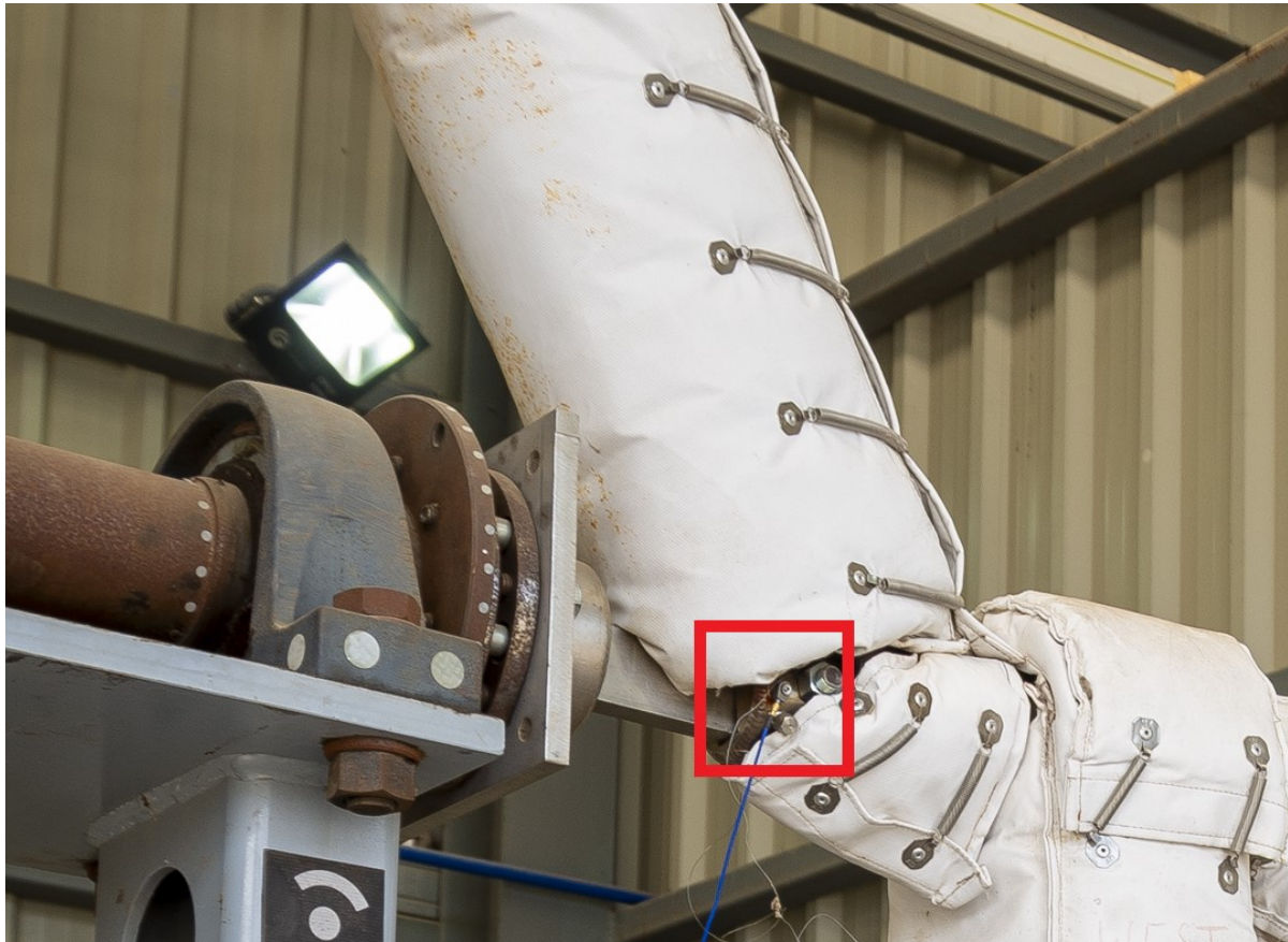
Figure 3.4: RFHA with installed vibration sensor (marked with red square)
