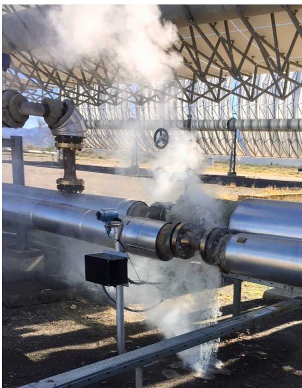
Fig. 14. HELISOL ® 5A leaking from flow meter flanges at 240 °C and 24 bar during solar operation, the thermal insulation was removed prior to the incident.
