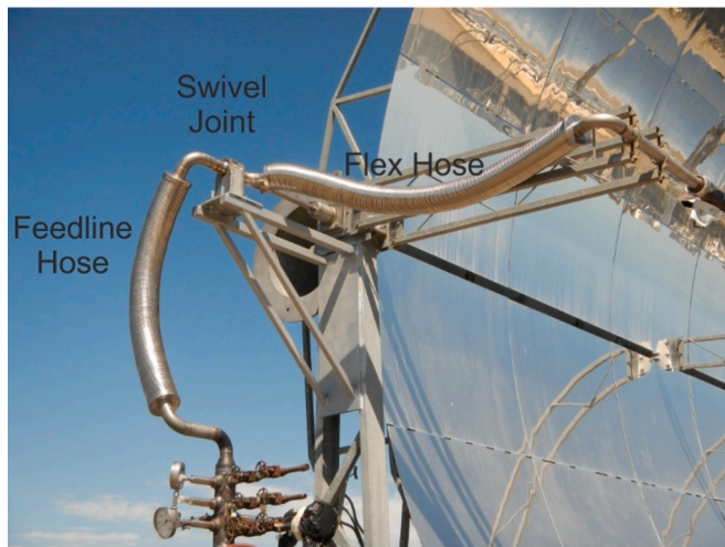
Fig. 3. Installed REPA (feedline hose, swivel joint and flex hose) at PROMETEO, thermal insulation not installed.
