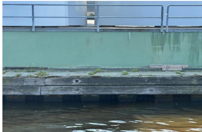
Fig. 5: Harbor quay with concrete bulwark and wooden planking. The bulwark is protruding 1.8m from the charted quay wall.
