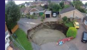
Voids leading to sinkholes
