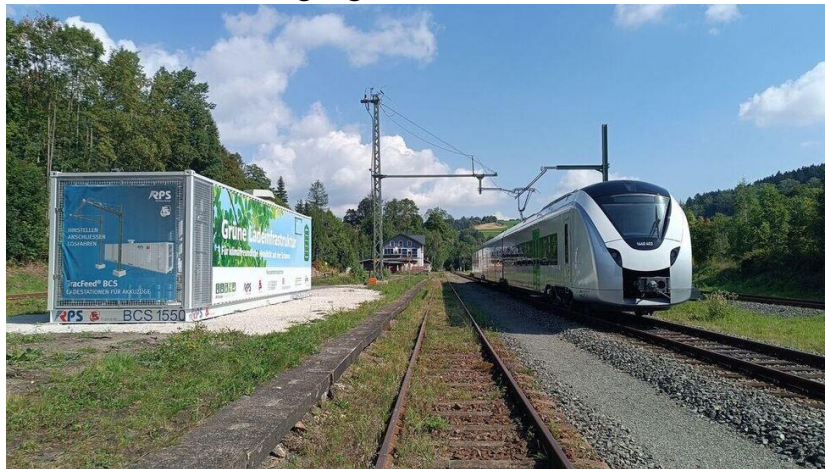
RCS BEMU Charging Station: 1.2 -2 MW
