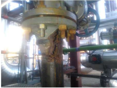
Molten Salt Corrosion in Chemical Boilers, Source: https://www.chemicalboiler.com/forensicengineering/molten-salt-corrosion/
