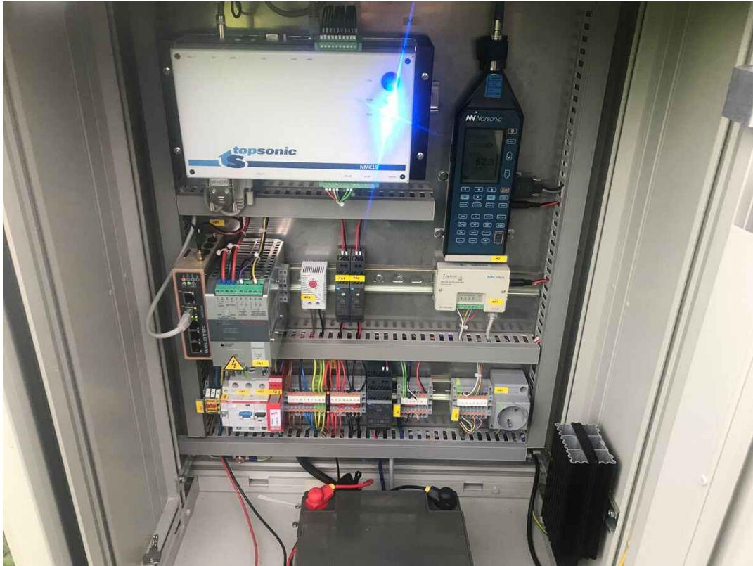
Figure 4.5.: Inside view of the Noise Monitoring Terminal (NMT). Hamburg airport employs the TANOS management system from the company Topsonic. The photo shows the technical equipment in figure (4.4). The equipment is used to save and transfer the data to the central data management system of the airport. It consists of a router, sound level meter, fuses, and a battery in case the electricity goes out.
