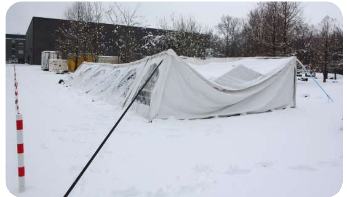
Collapse of outdoor tent after snowfall event
