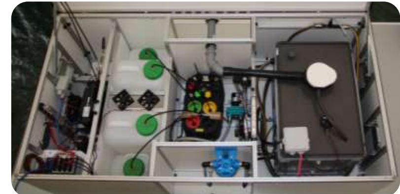
ASU inside view during 1st outside test
