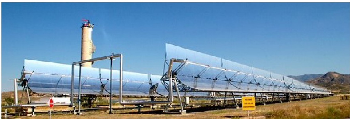
Fig. 4.24: Picture of the Parabolic Trough DISS at CIEMAT'S PSA. The tower of the CESA-I power plant can be seen in the background [73].
