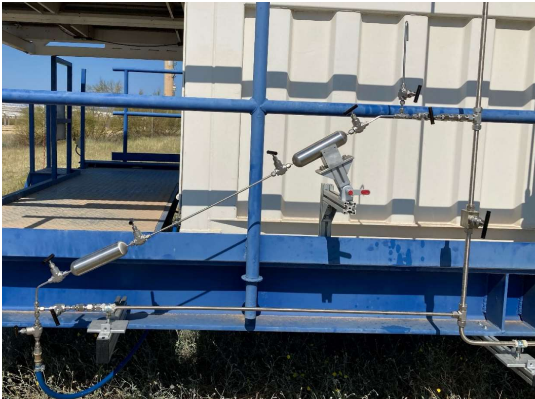
Figure 22: Close up of the HTF sampling station (prior to the installation of thermal insulation)
