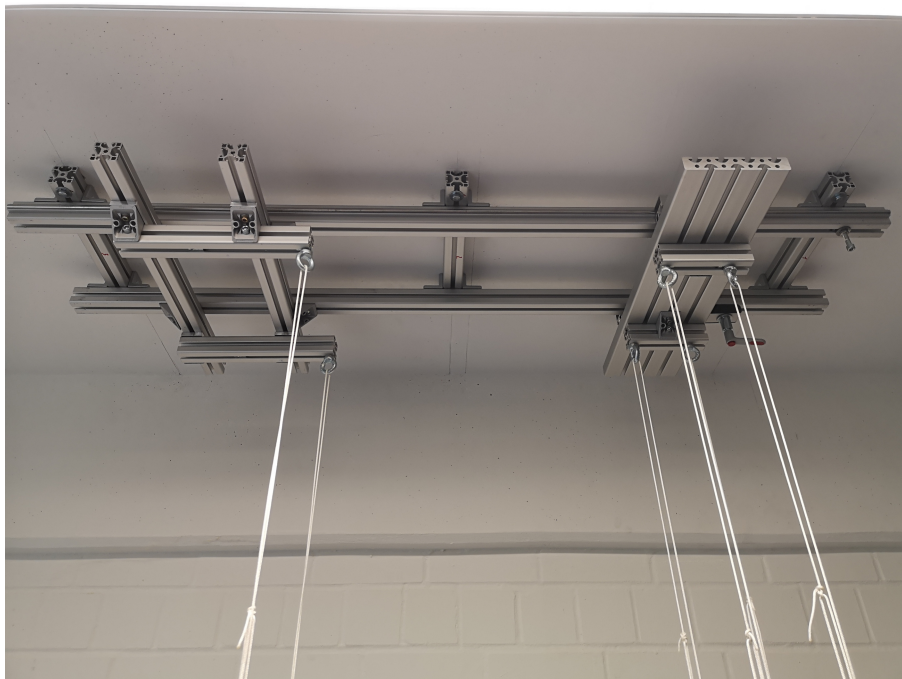
Figure 20: Ceiling mounting structure at LET Laboratory.
