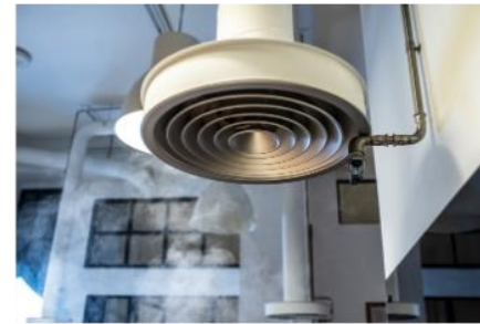
Advanced & recycling ventilation system
