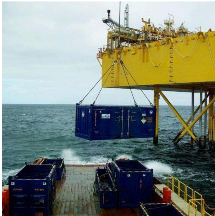
Figure 6- DEPICTS THE TRADITIONAL CRANE METHOD FOR TRANSFERRING THE CONTAINER TANKS TO VESSEL (wilson son)
