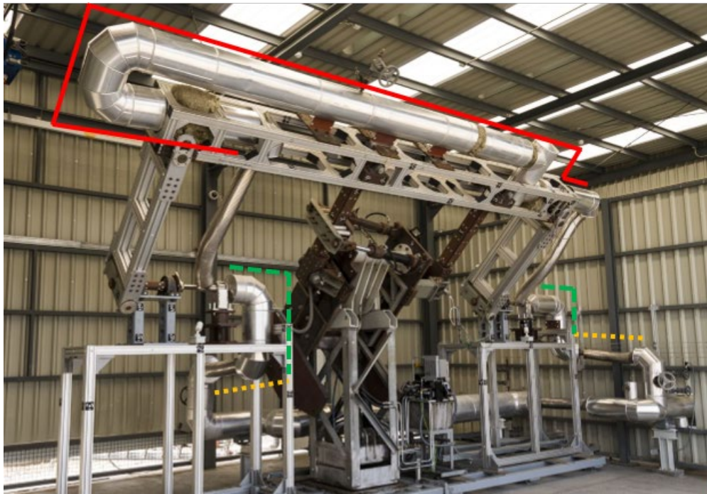
FIGURE 1. Overview of the kinematic unit with two flex hose assemblies mounted, left east, right west solid red line: indicating the moving tube section, green dashed line: indicating the bottom connections to both REPAs under testing, yellow dotted line: indicating the orientation of the flex hoses as part of the bottom connection
