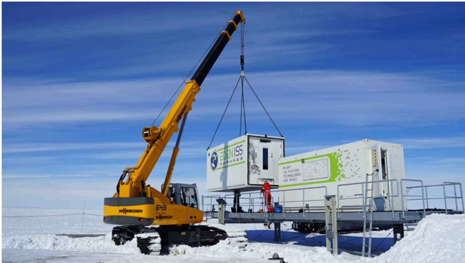
Installing the EDEN ISS containers on the platform (400m away from the station).
