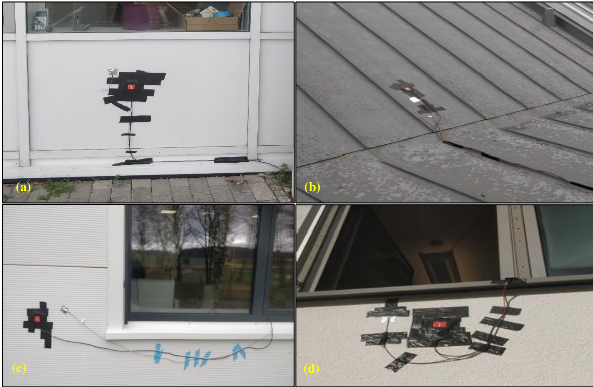
Figure 8. Heat flux sensors and temperature sensors installed at different places within the building. (a) block A outside PVC wall, (b) block D outside roof, (c) block E outside PVC wall, (d) block D outside plaster wall.
