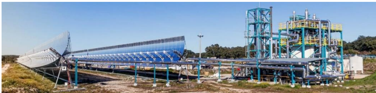
Fig. 1: Side view of the molten salt parabolic trough collector and storage system at Évora Molten Salt Platform. (Credit: University of Évora / Hugo Faria).
