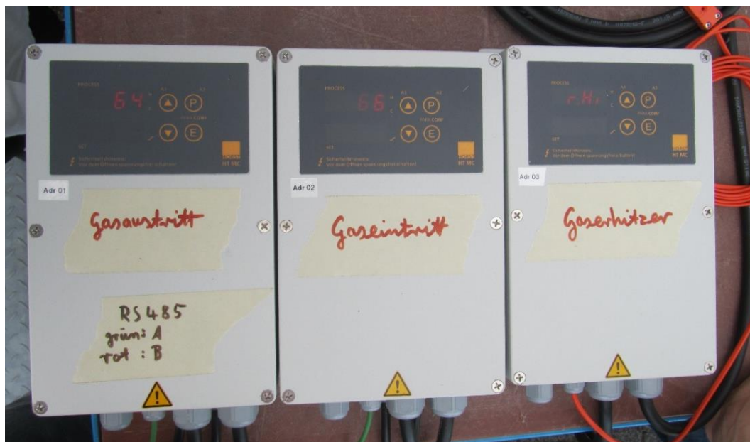
Figure 3.10 Control boxes for heating elements from Horst
