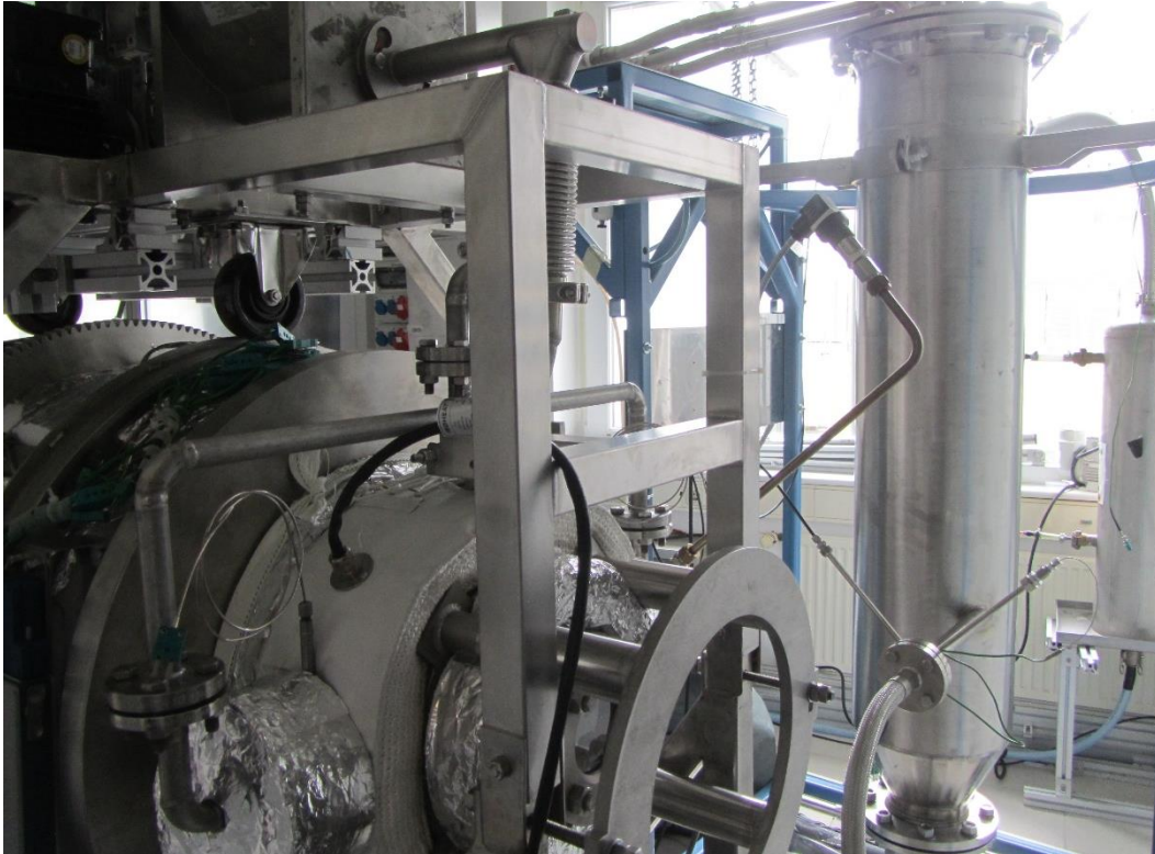
Figure 3.13 Carbonator connected to the filter unit
