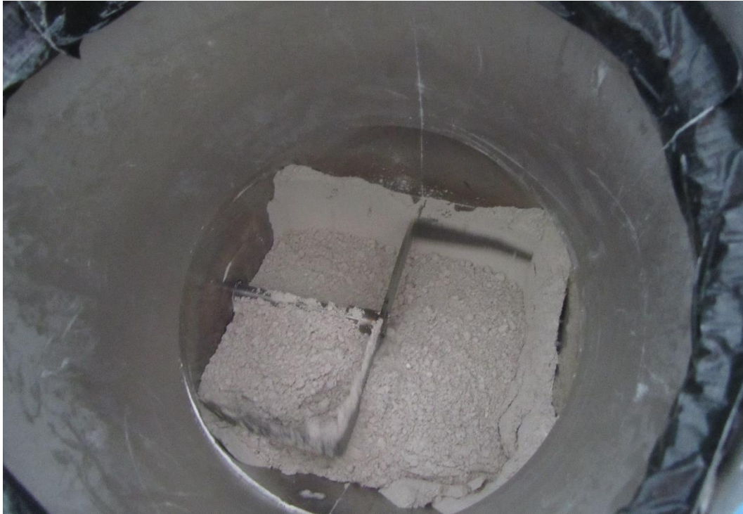
Figure 5.5 Inside of the screw feeder (bridge breaker)
