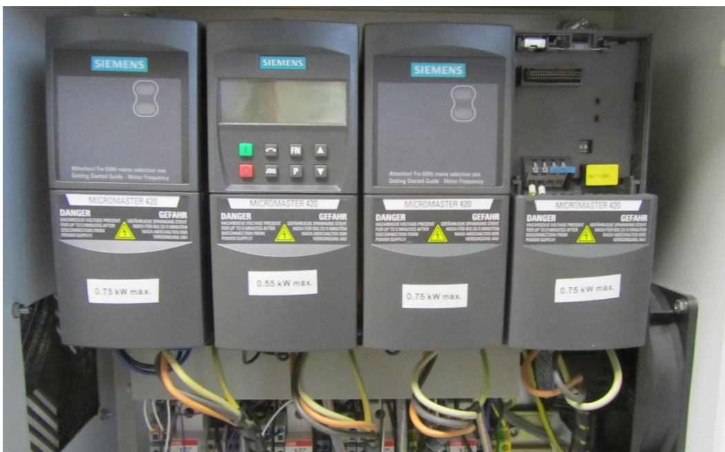
Figure 3.6 Siemens Micromaster 420 Frequency converters
