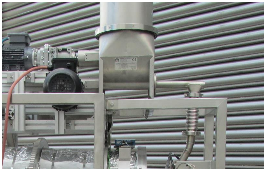
Figure 3.7 Flexible connection of screw feeder and reactor
