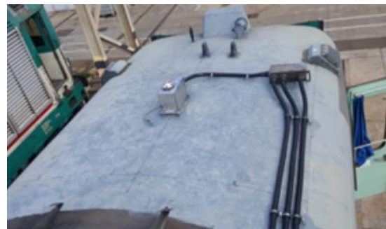
Figure 2. Antenna installation, Italy.
