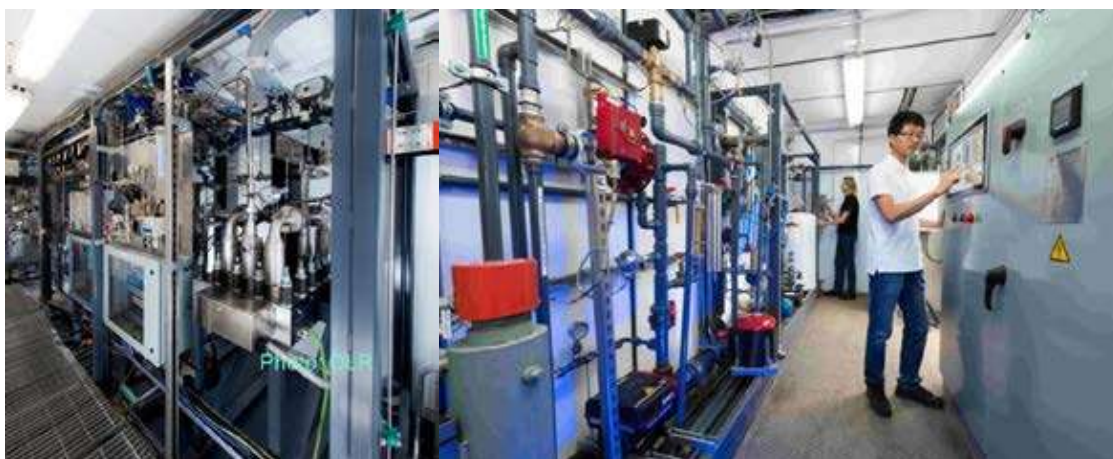
Fig. 2: process room (left) with stack and operation room (right) with HMI (Human machine Interface) and DI water processing of 50 kW experimental electrolyser used at DLR
