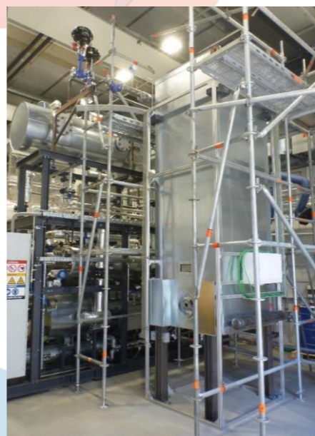
Testing: 160 kWh unit designed, built and currently in testing phase
