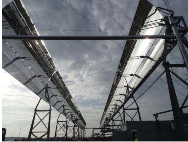
FIGURE 3. Parabolic trough collectors for steam generation at ADPO plant in Belgium
