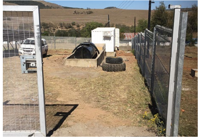
Figure 30: Minigrid fenced area
