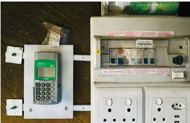
Figure 27: Ready board installed at the household (electricity outlets and payment system)
