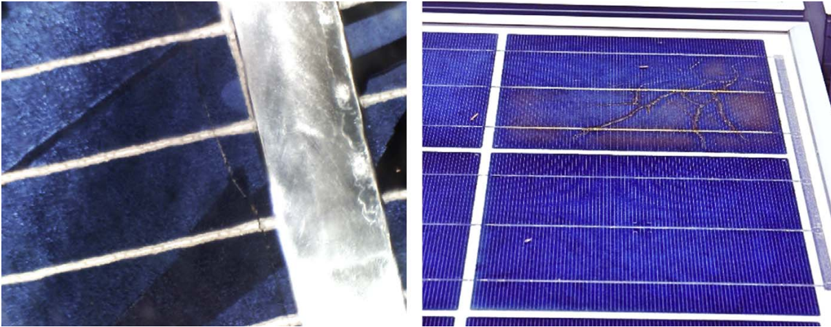
Figure 2.8: Cases of cell cracks (left) and consequent snail trails effect (right) in two different PV modules. [4]
