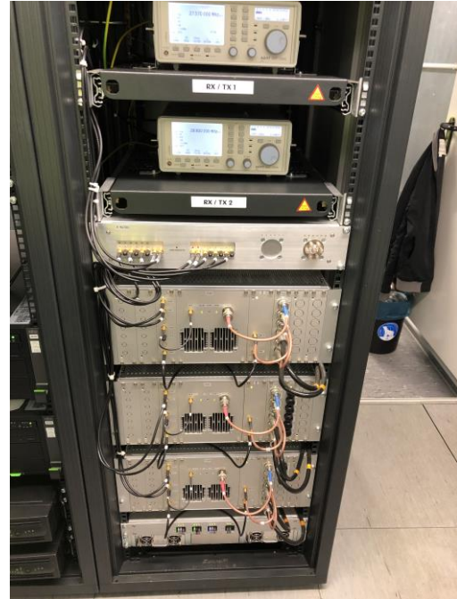
Fig. 7. RF rack. From top to bottom: redundant transceivers, switching matrix, VHF/UHF/S Band frontends, PSU
